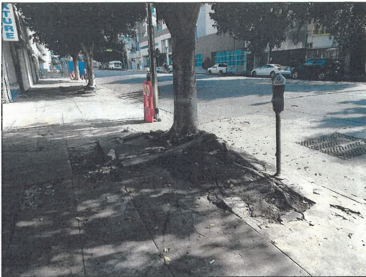
Extensive surface roots from ficus tree no. OS-3 that are causing destructive damage to surrounding sidewalk and city hardscape.
