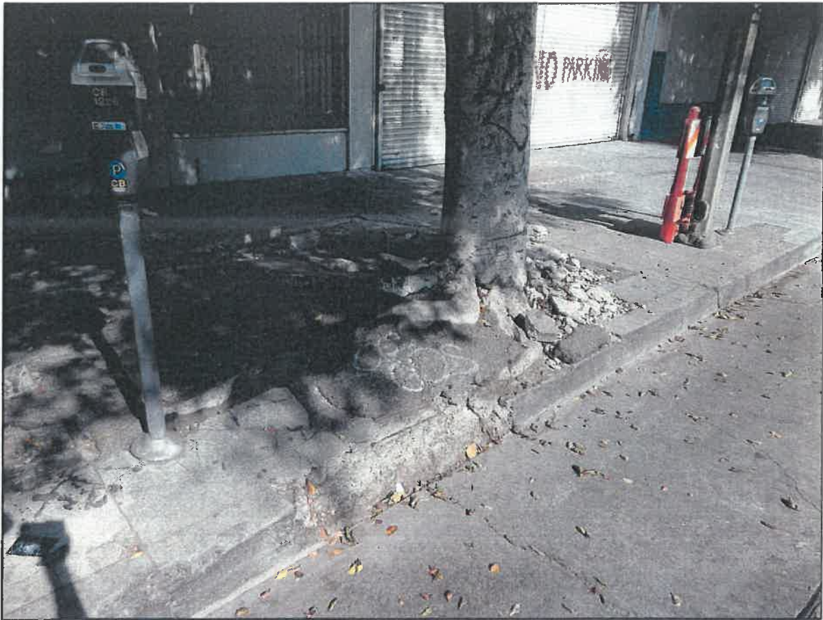
Extensive surface roots from ficus tree no. OS-3 that are causing destructive damage to surrounding sidewalk and city hardscape.
