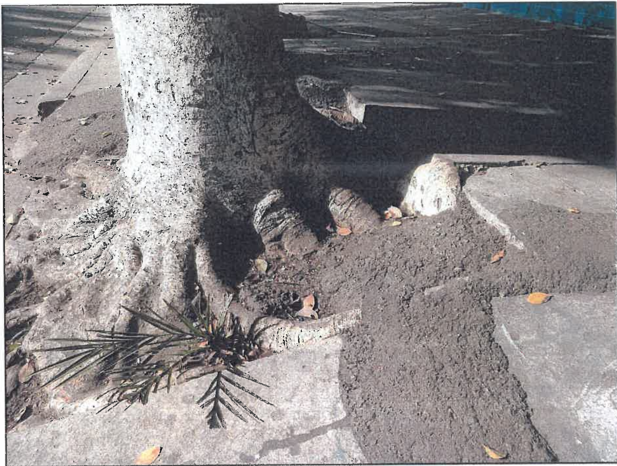
Extensive surface roots from ficus tree no. OS-2 that are causing destructive damage to surrounding sidewalk and city hardscape.
