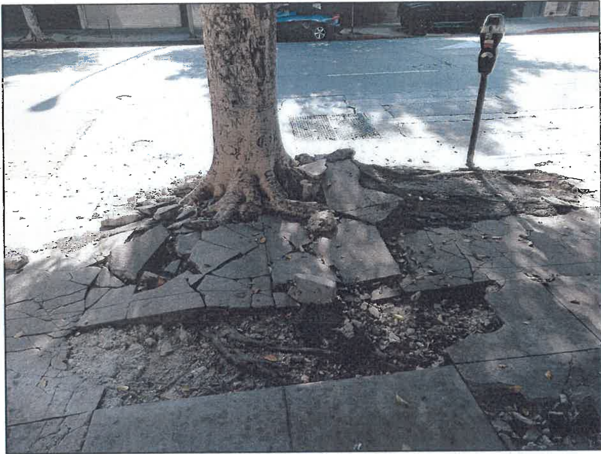
Extensive surface roots from ficus tree no. OS-3 that are causing destructive damage to surrounding sidewalk and city hardscape.
